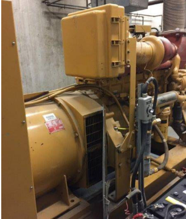
Example 33. Indoor Generator
