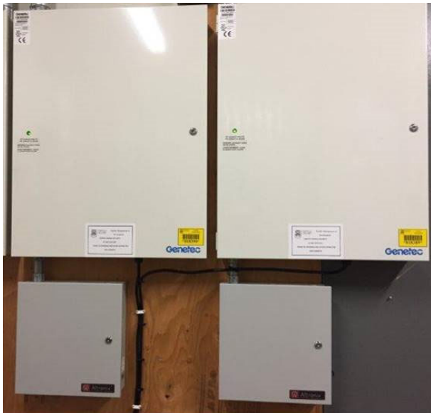
Example 31. Door Access Panels
