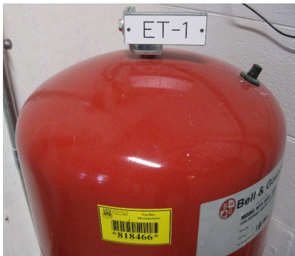
Example 15. Expansion Tank
