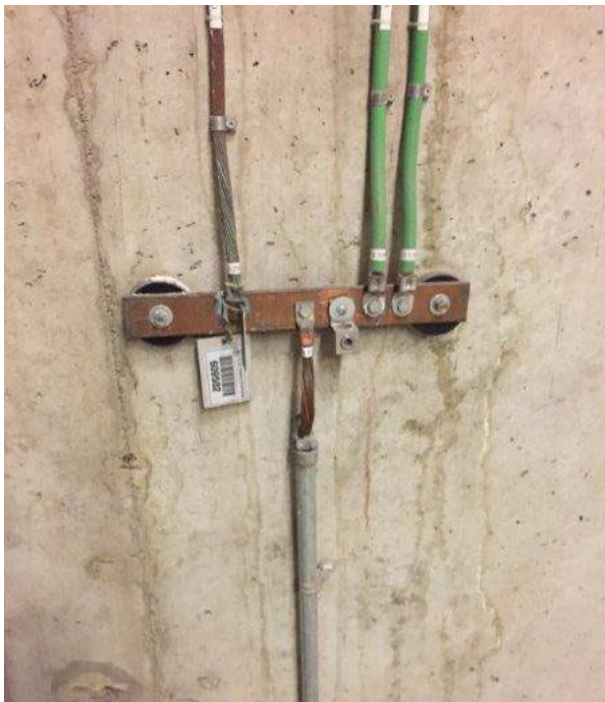
Example 35. Main Electrical Distribution Ground Bar
