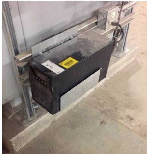
Example 40. Controls UPS
