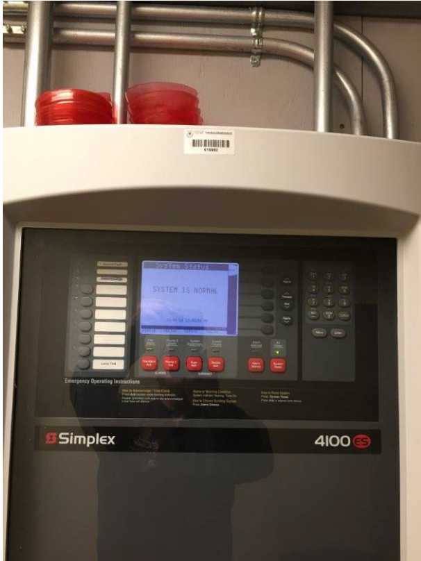
Example 21. Fire Alarm Panel
