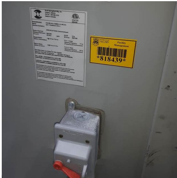
Example 1. Air Handling Unit
