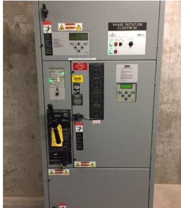
Example 34. Transfer Switch
