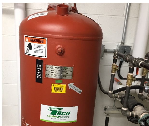
Example 16. Expansion Tank
