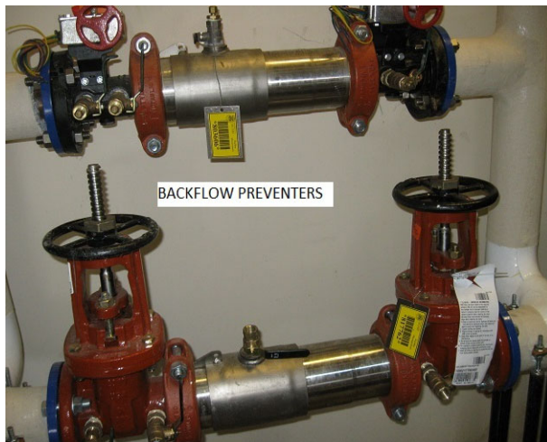
Example 3. Backflow Preventors
