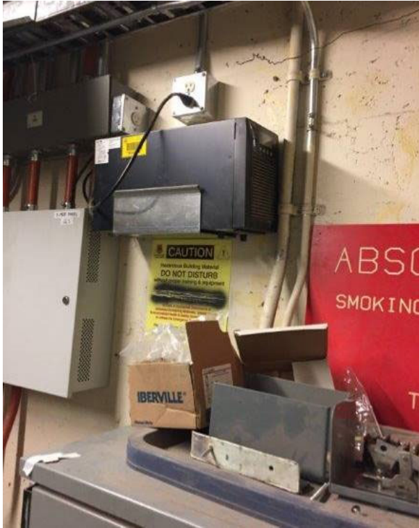
Example 41. Controls UPS
