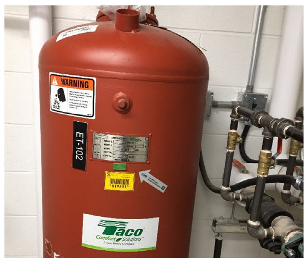
Example 16. Expansion Tank
