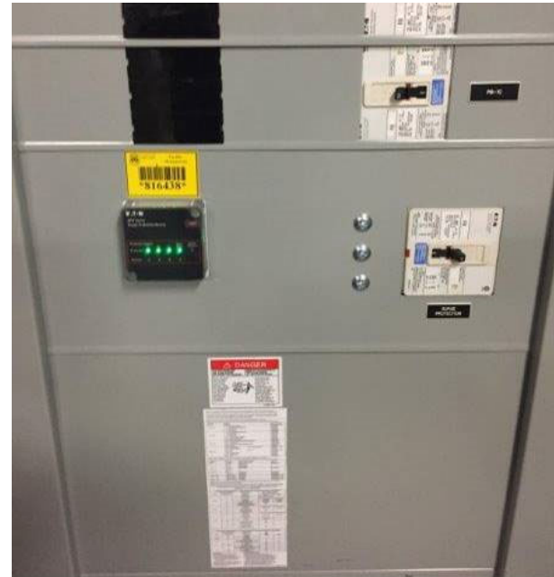
Example 44. Surge Protection Device
