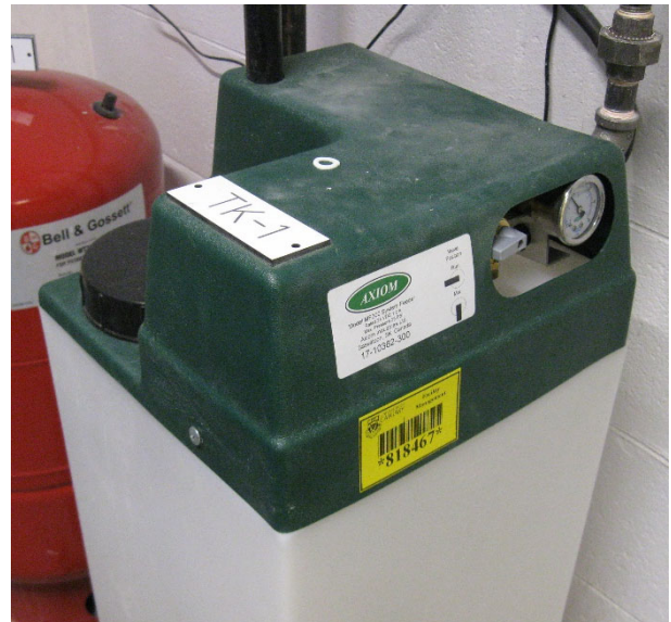
Example 12. Glycol Feed Tank
