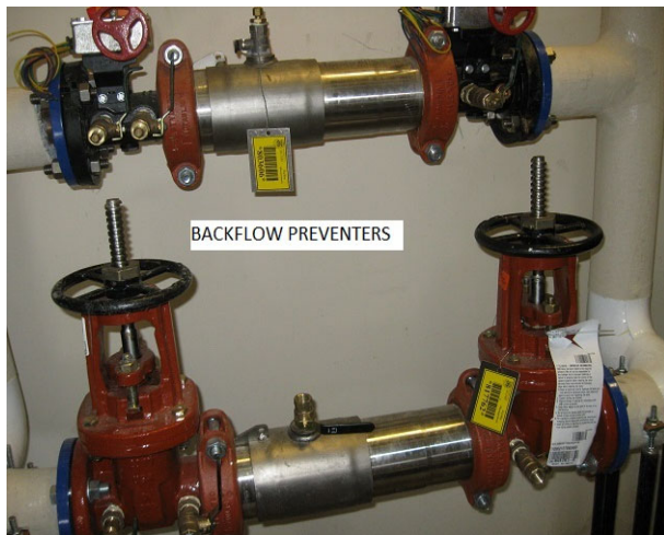
Example 3. Backflow Preventors
