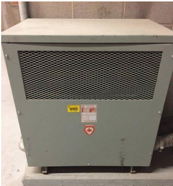
Example 39. Low Voltage Transformer
