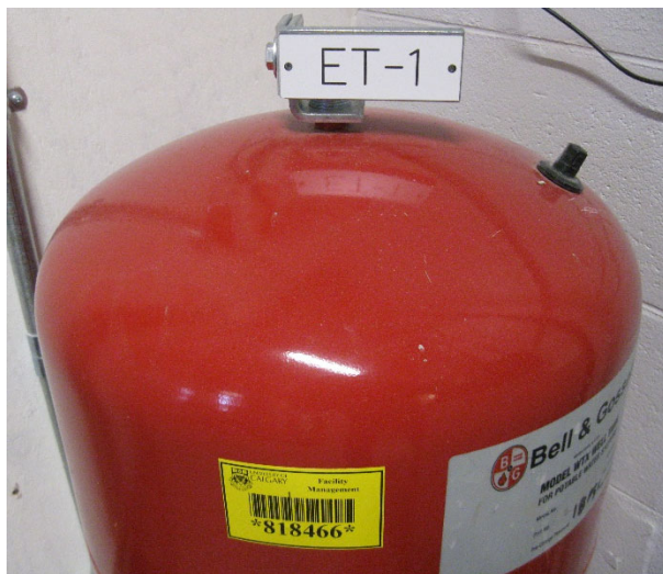
Example 15. Expansion Tank
