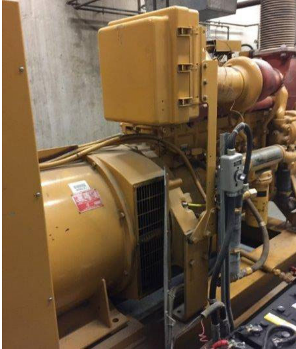
Example 33. Indoor Generator
