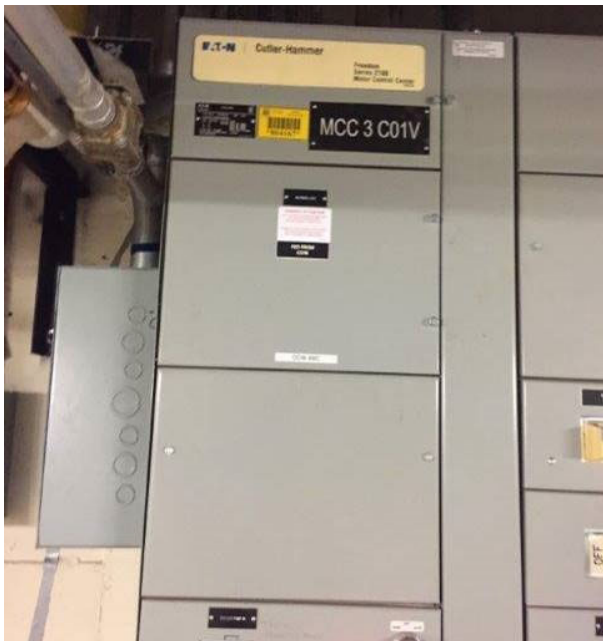
Example 43. Motor Control Center
