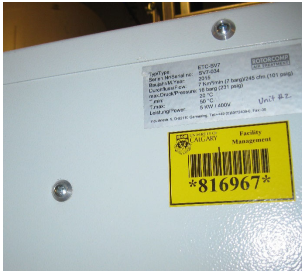
Example 5. Air Compressor
