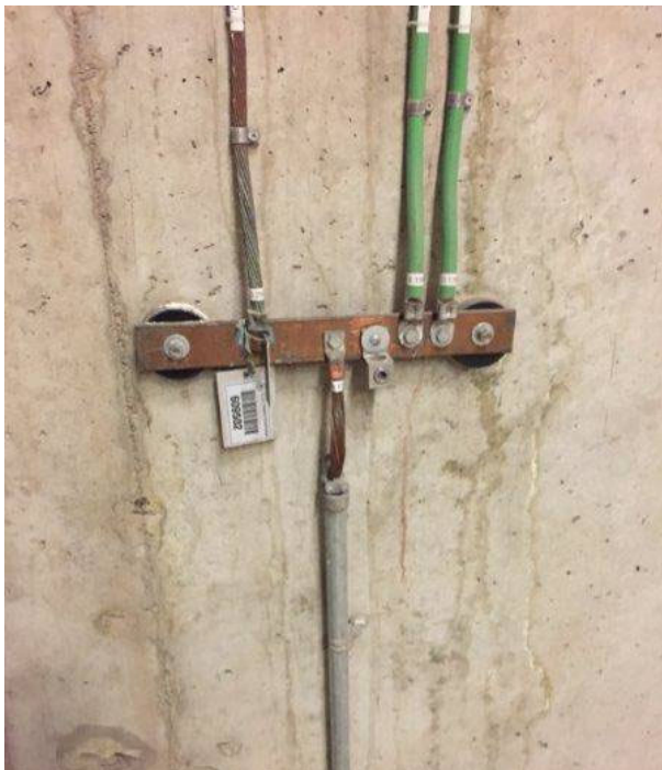
Example 35. Main Electrical Distribution Ground Bar
