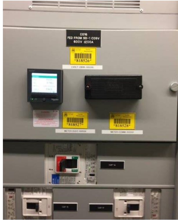
Example 42. Electrical Utilities Metering
