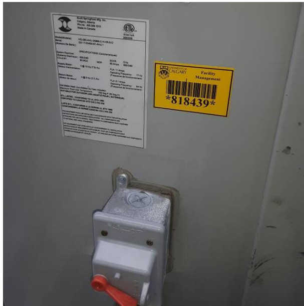
Example 1. Air Handling Unit
